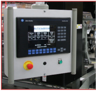
Allen-Bradley PanelView controls
